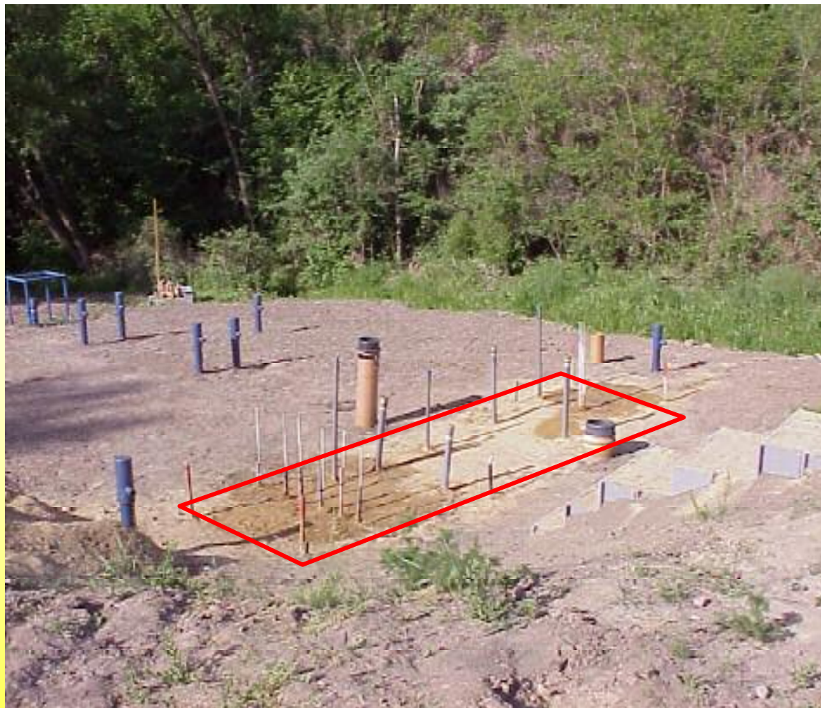
View of the experimental permeable reactive barrier with monitoring wells (Csővári et al.)
